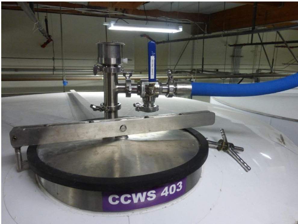
Closed top fermentation tank with EcoPAS piping
