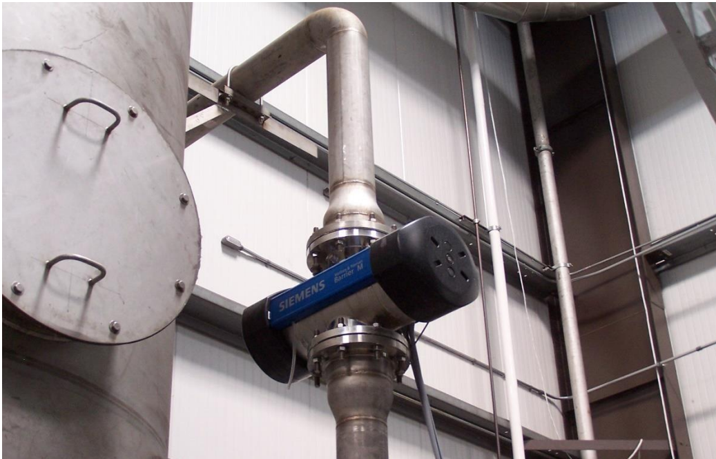
Packed bed scrubber and UV treatment lamp
