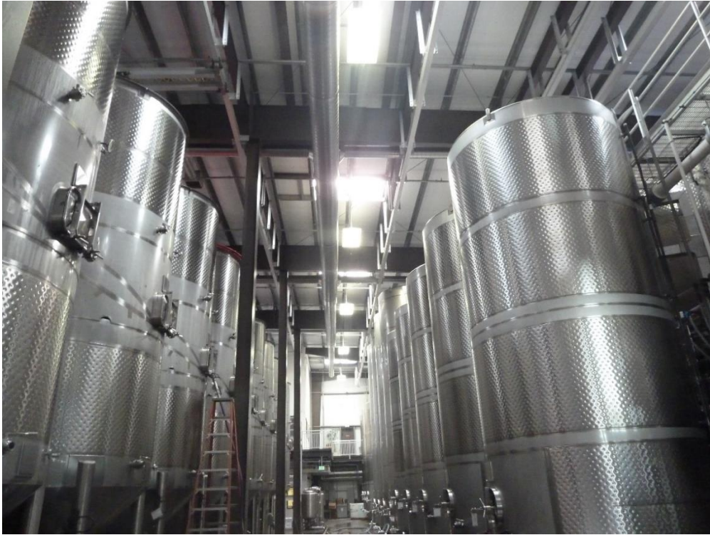
Wine fermentation tanks and fermentation room ventilation ducting
