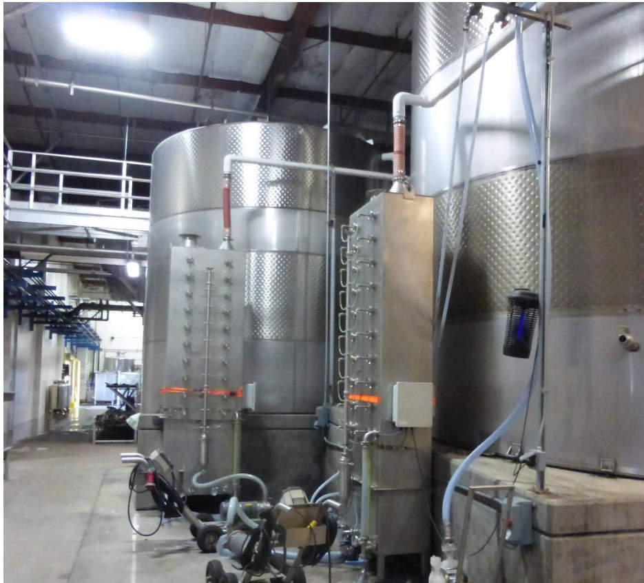
NoMoVo control systems (2)
