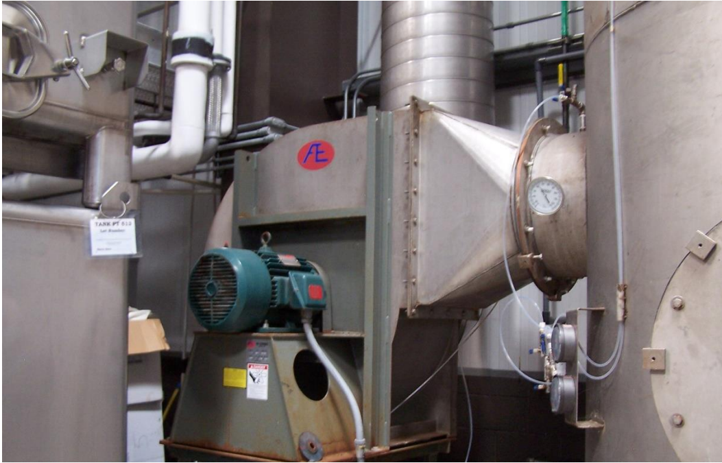
Packed bed scrubber blower
