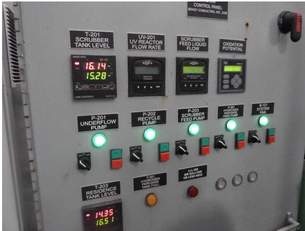
Packed bed scrubber control panel
