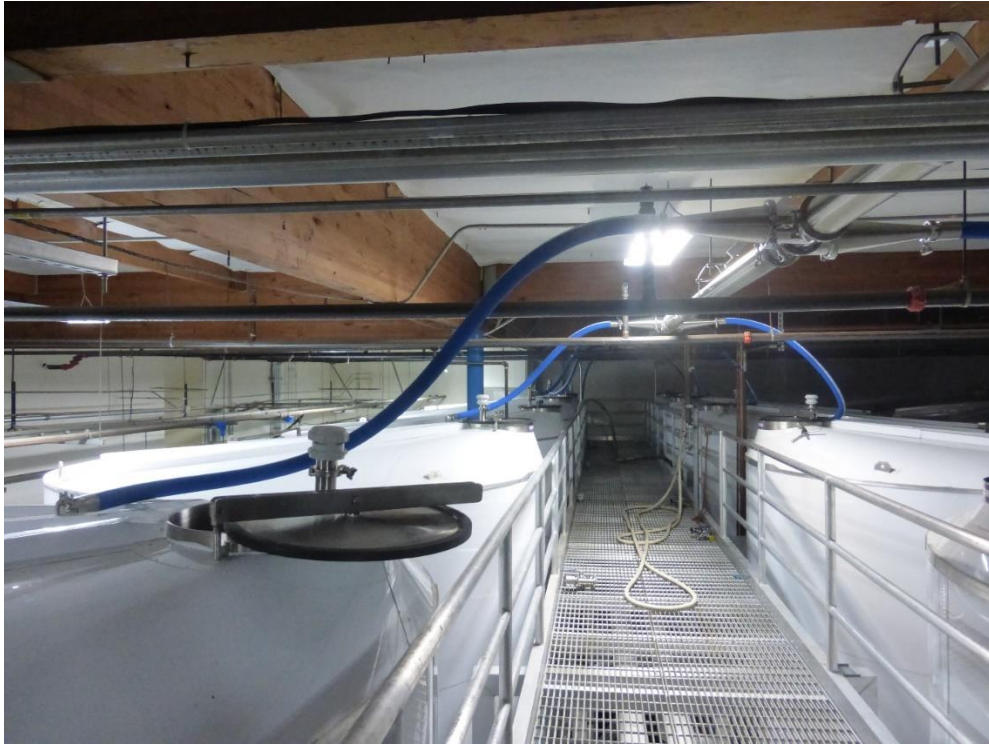
Closed top fermentation tanks with EcoPAS piping manifold
