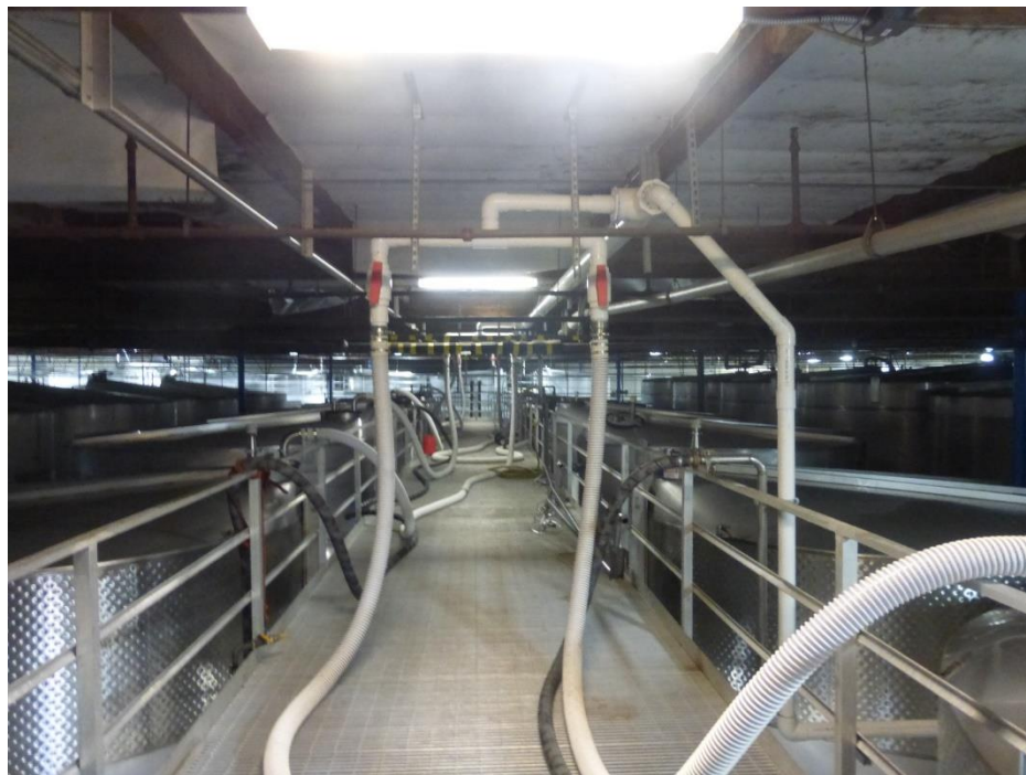
Closed top fermentation tanks with NoMoVo piping manifold
