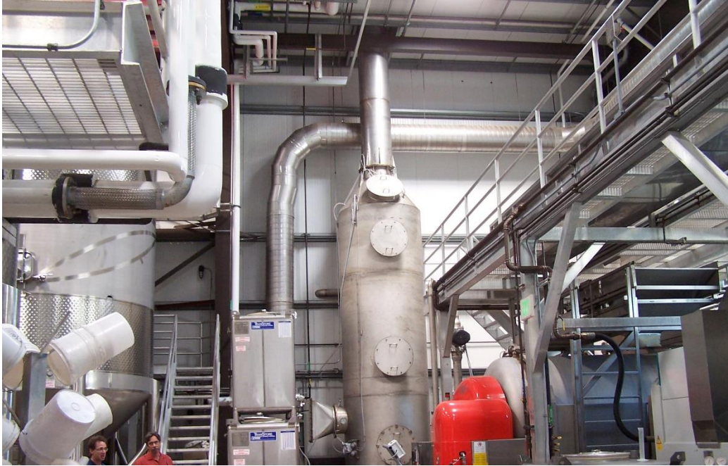
Packed bed scrubber
