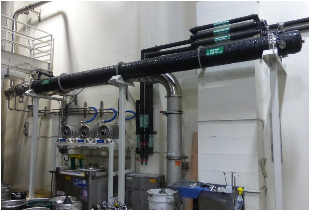
EcoPAS control system
