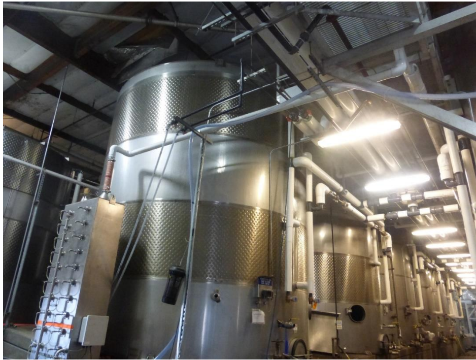
NoMoVo control system with NoMoVo piping manifold
