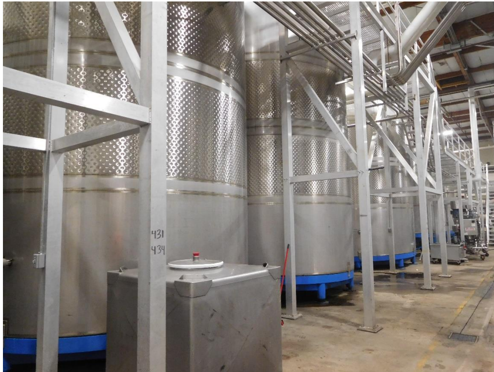
CCWS Series 400 tanks and EcoPAS piping manifold
