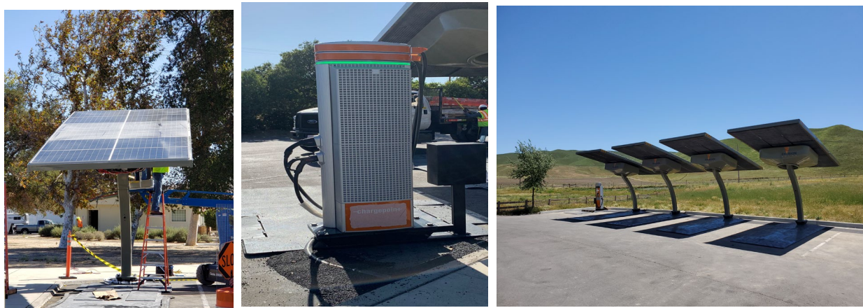
Photos of solar-powered electric vehicle stations at Camp Roberts and Shandon Rest Areas.
